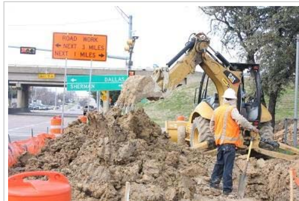
Dan Eakin/Staff Photo - Workers remove dirt at the northeast corner of U.S. Highway 75 (North Central Expressway) and Louisiana Street in McKinney. Work crews began moving dirt this week in order to relocate utilities in preparation for the widening of U.S. 75 between Sam Rayburn Tollway and U.S. Highway 380.
